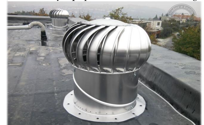
Ventilation turbine built on a roof of an apartment building (Lomanco BIB 14)
