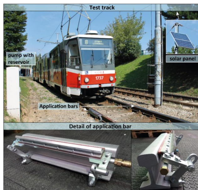
Fig. 5.6 Detail of wayside lubrication system.
